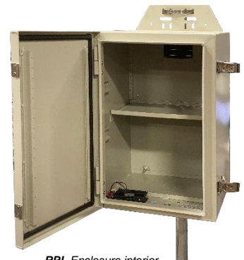
RPL Enclosure interior without batteries or controller
